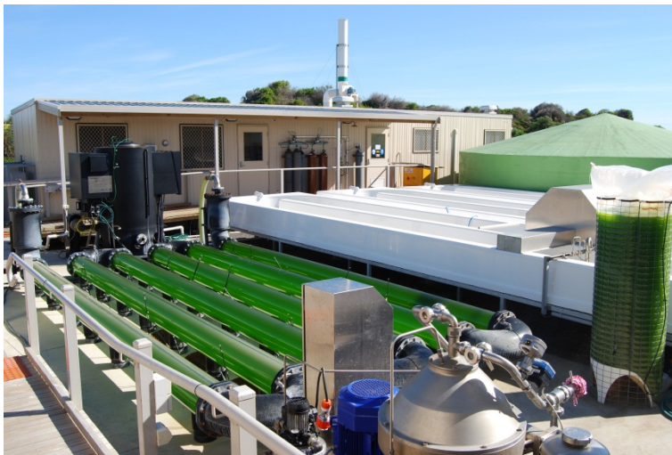
Figure 14. SARDI Aquatic Sciences: the NCRIS Photobioreactor Facility
