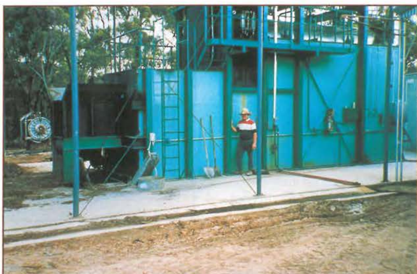
A 300 hp colonial boiler with Dutch oven for burning extracted leaves
